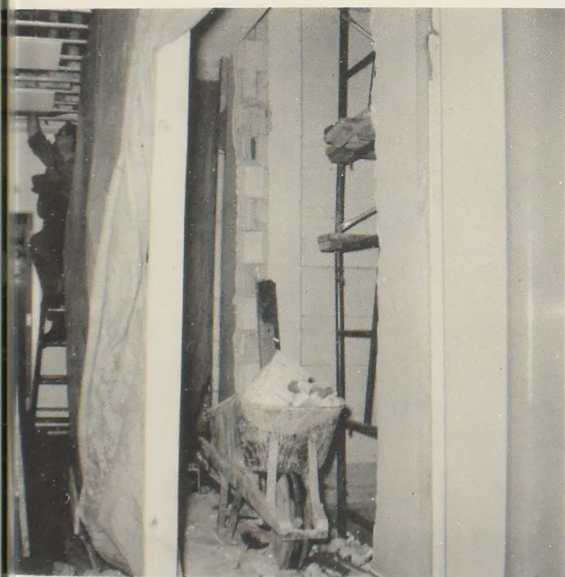
New Elevator Shaft
